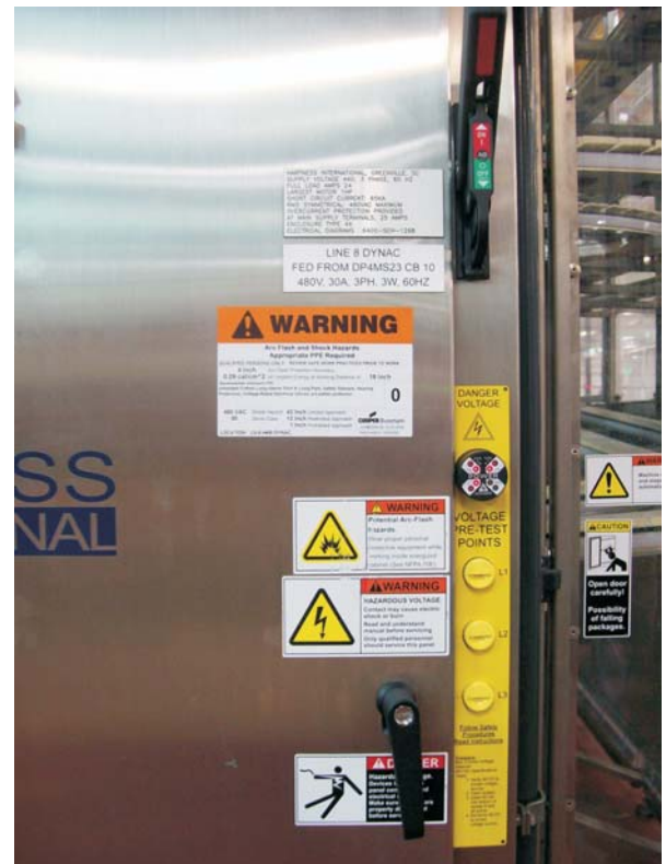
Fig. 6 Installation of a voltages indicator and voltage portals on a typical 3-phase panel.
