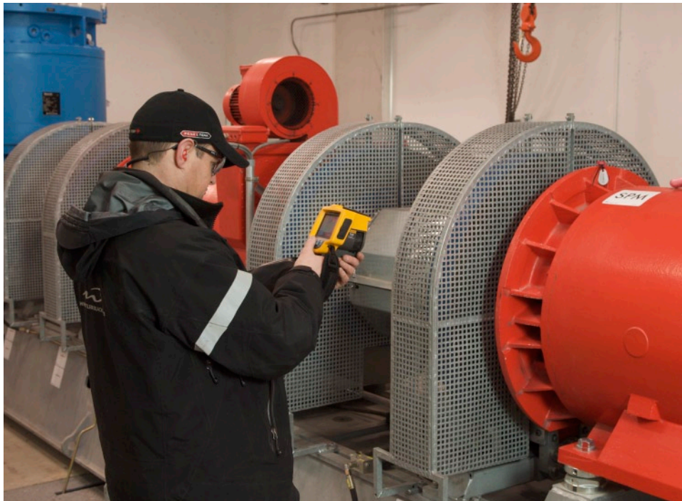
Rob Withey uses a Fluke thermal imager to check temperature on bearings and gearbox housings on the 335 kW (450 hp) motors in the Peak 2 Peak main drive room.
