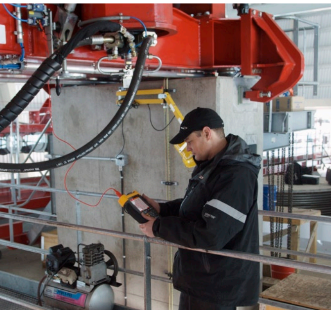
The Whistler/Blackcomb Peak 2 Peak gondola has many safety and redundant electrical systems. Rob Withey uses a Fluke ScopeMeter to look for voltage drop at a switch.
