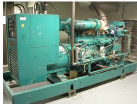
A 300 kW Cummins Power Generation standby generator provides backup power and now also powers the pumps during peak demand periods.
