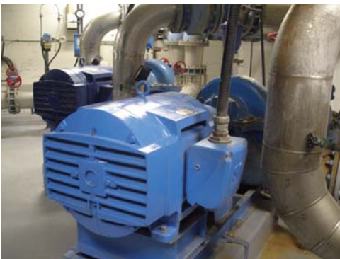
Two large pumps supply water to a hilly part of the service area. Using the standby generator to power them during the utility's peak demand period reduces strain on the grid.
