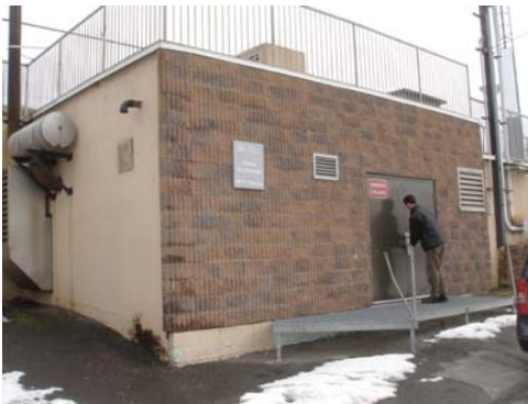
A critical Hydro Sherbrooke pumping station was chosen to test the new closed-transition transfer switch during load-shedding.
