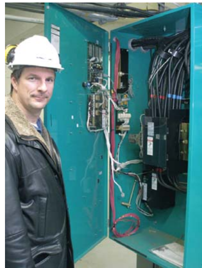
Hydro Sherbrooke's Pierre Frechet inspects the new closed-transition transfer switch.
