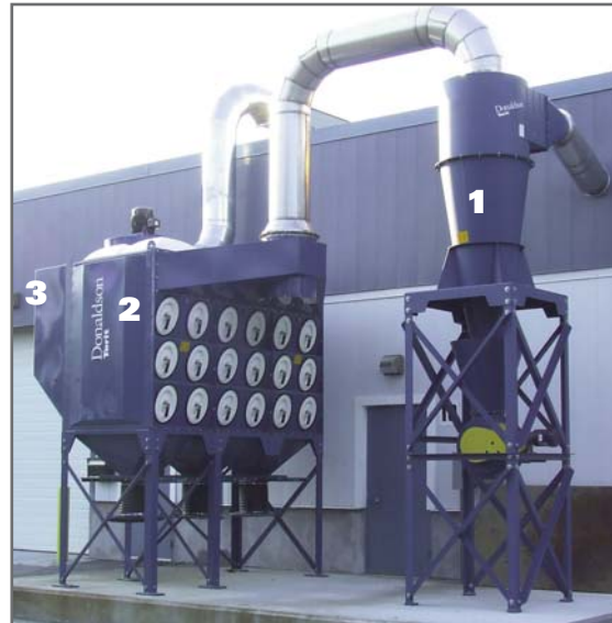
The new state-of-the-art spray booths at Falmer Thermal Spray (Salem, MA) are ducted outside the building into a (1) Donaldson Torit cyclone pre-cleaner, (2) then into Downflo Oval (DFO) dust collector with Ultra-Web® filters, and (3) finally through a HEPA filter. The system controls hexavalent chromium and other particulate from the daily operations.
