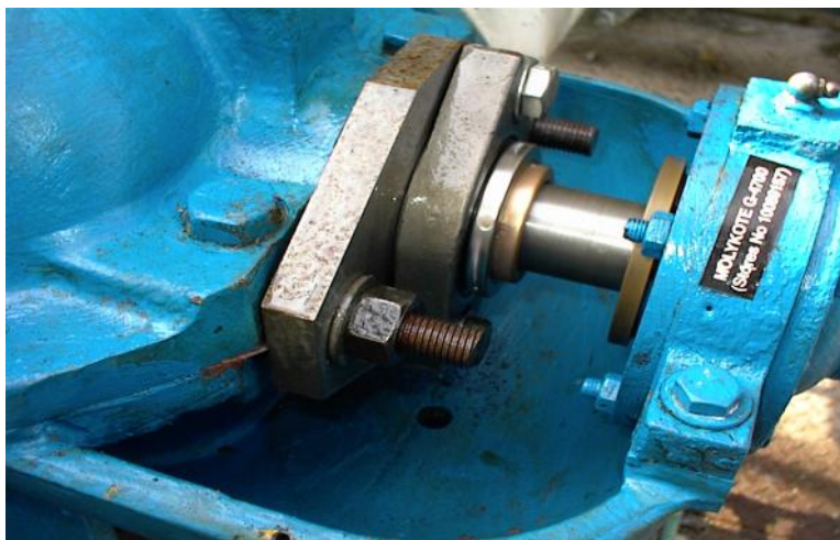
Figure 3: New Mechanical Seals Eliminated Leakage
